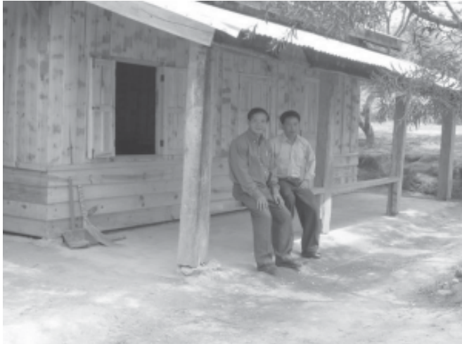
Completed 2008 project—rebuilt life-skills school building ready for school to open at Ban Phosy.
