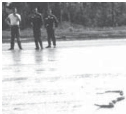
The hot emulsified asphalt attracted snakes and other animals in the early evening because it was warm and felt good as the temperature started to fall towards nightfall. The asphalt set up as it cooled and the snakes and other animals were caught in it like this cobra. The longest snake caught at NKP was an eight foot spitting cobra. (May 1963)
